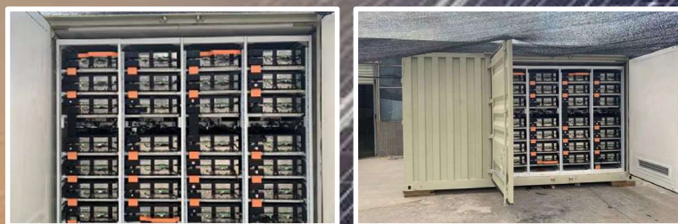
1 MWh Energy Storage System
